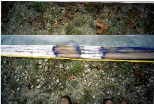
Stains on cover in 3" cored hole
